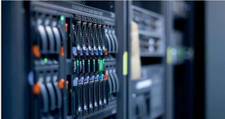
GALILEO CONNECT LONDON CENTRAL 2012 London (Great Britain) Application: Data Center Plant type: HPAC System
