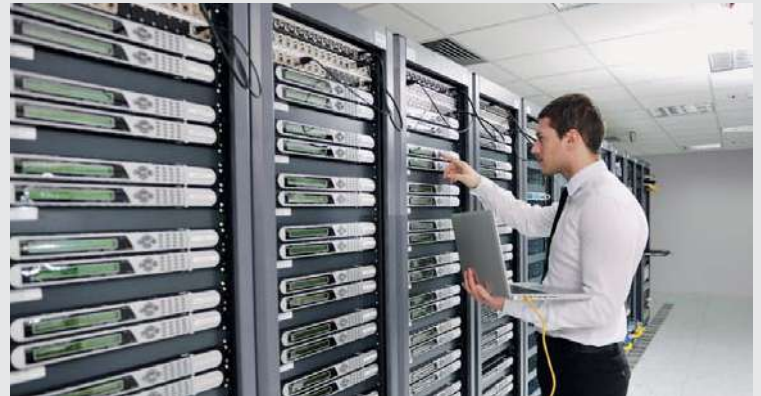
TELECOM DATA CENTER ACILIA, TIER IV 2016 Rome (Italy) Application: Data Center Plant type: Hydronic System
