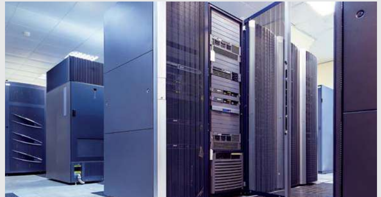
FASTWEB DATACENTER, TIER IV 2014 Milan (Italy) Application: Data Center
